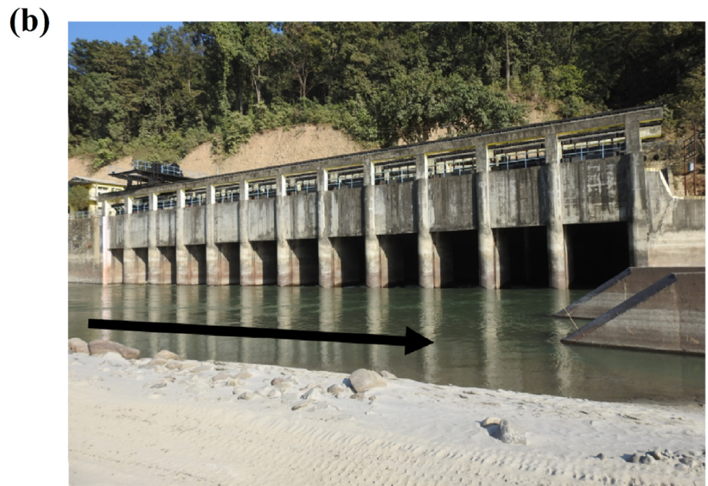
Figure 6. Headwork intake structure (12 rectangular orifices) of the Sunsari Morang Irrigation Scheme in the Koshi River (a) during the monsoon season, and (b) during the dry season (arrow shows the direction of river flow).
